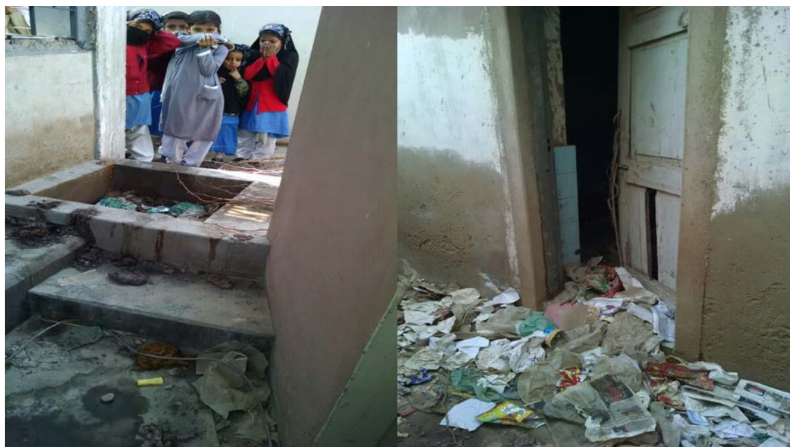
Toilet condition in Urban School
